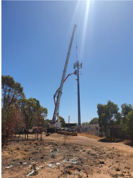
Photograph 5: View of crane on the site working on a mobile tower near Douglas Street
